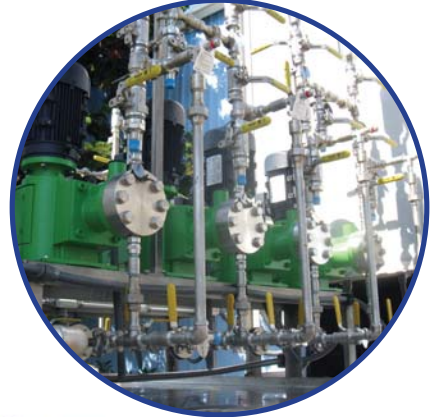
Phosphate Feed Skid
